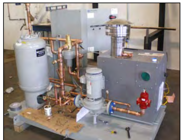
This boiler skid was prefabricated at the ACCO piping shop by Local 38 member Jason Hebbert.
