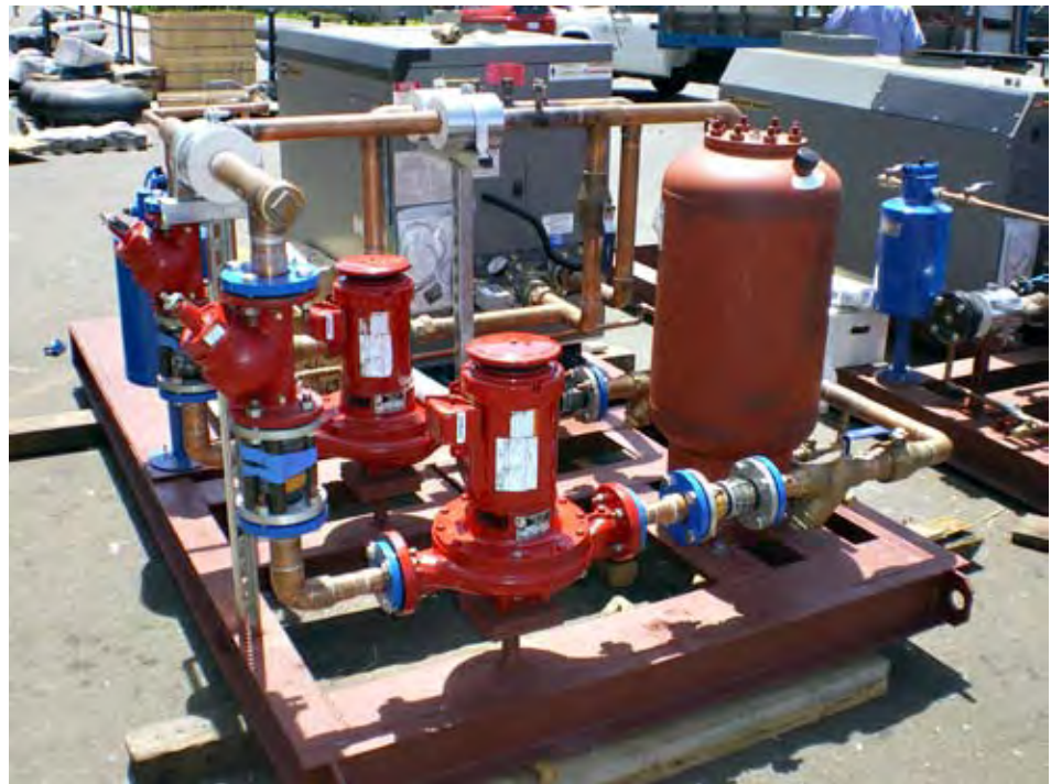
This pump skid is set to be installed at 150 Pacific St. in San Francisco. It was piped at the ACCO piping shop by Local 38 members Robert Reyes and Justin Furtado.
