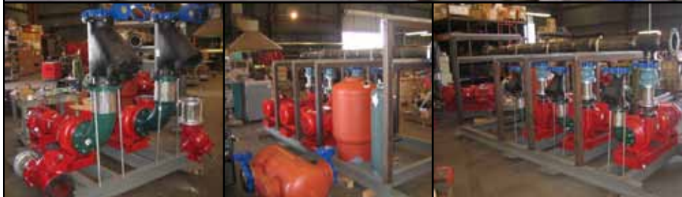
AR&B's have been able to prefabricate pump skids for their 200 Paul Street high-tech "digital real estate" facility, ensuring that the work remains with Local 38 members.
