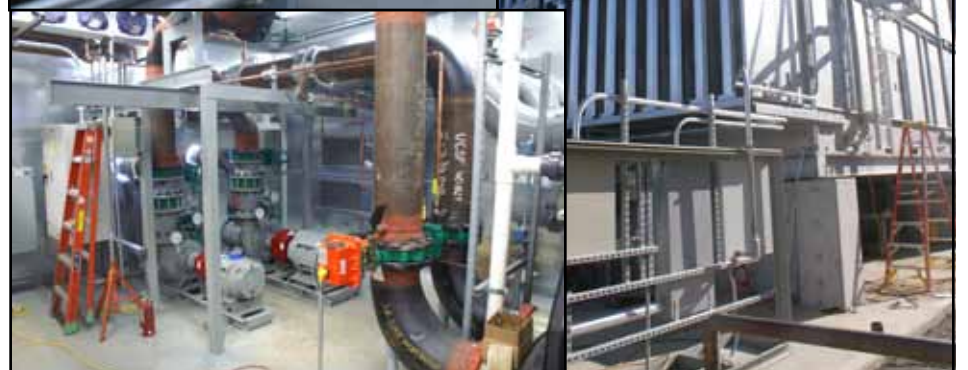
Southland Industries Preliminary Utility Plant (PUP) was prefabricated at their Union City shop by Local 38 hands, and then driven to the jobsite. The moving had to be done at night, so as not to disrupt traffic.
